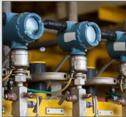
Instrumentation and Controls
