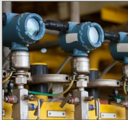
Instrumentation and Controls
